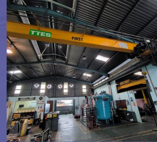
5-Tonnes Overhead Crane
