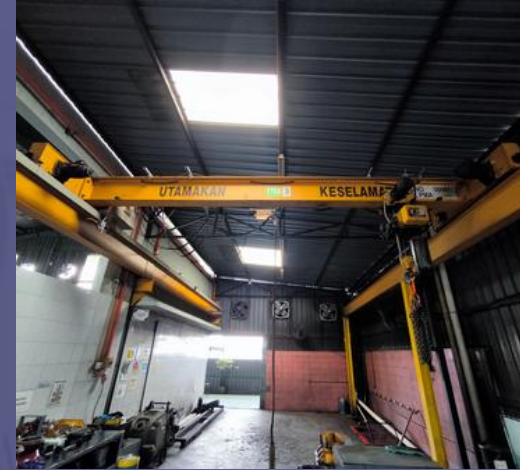
3-Tonnes Overhead Crane
